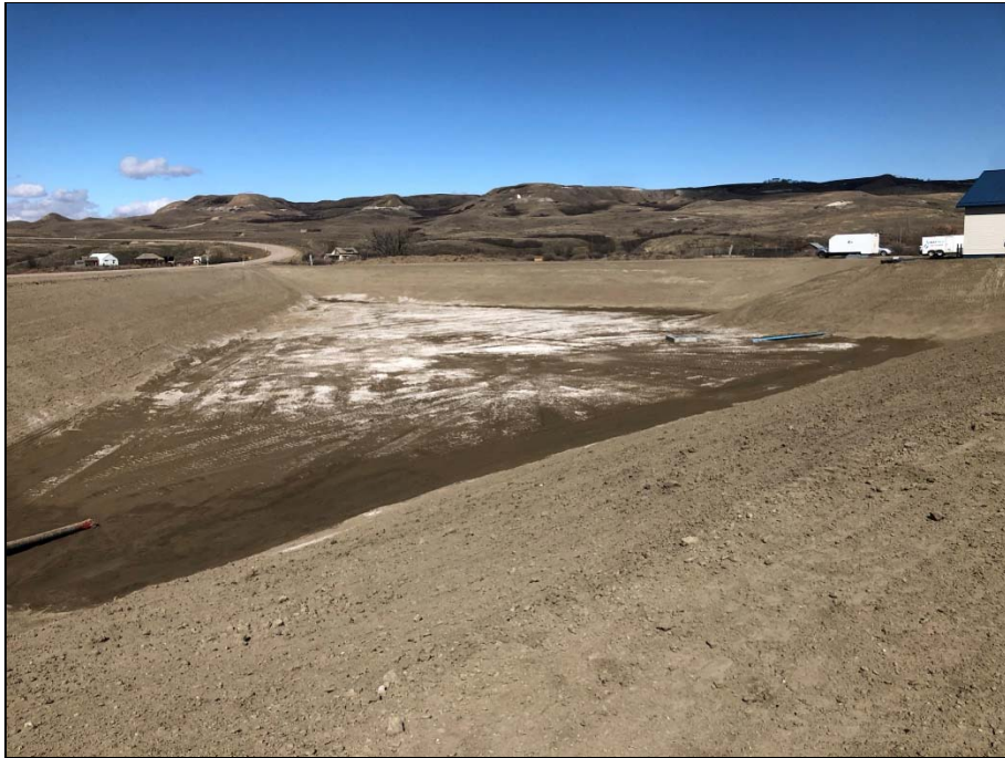
Reservoir floor is drying but requires additional geotextile and fill to firm up for liner install.
