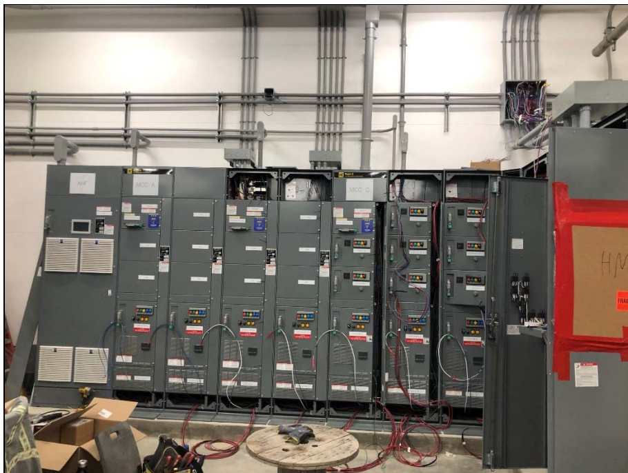
Motor control centre wiring (starters and variable frequency drives).
