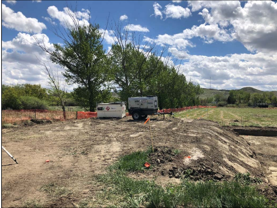
Generator and site perimeter fencing.
