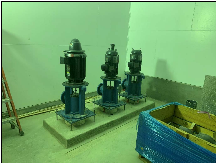
Transfer and backwash pumps are set.
