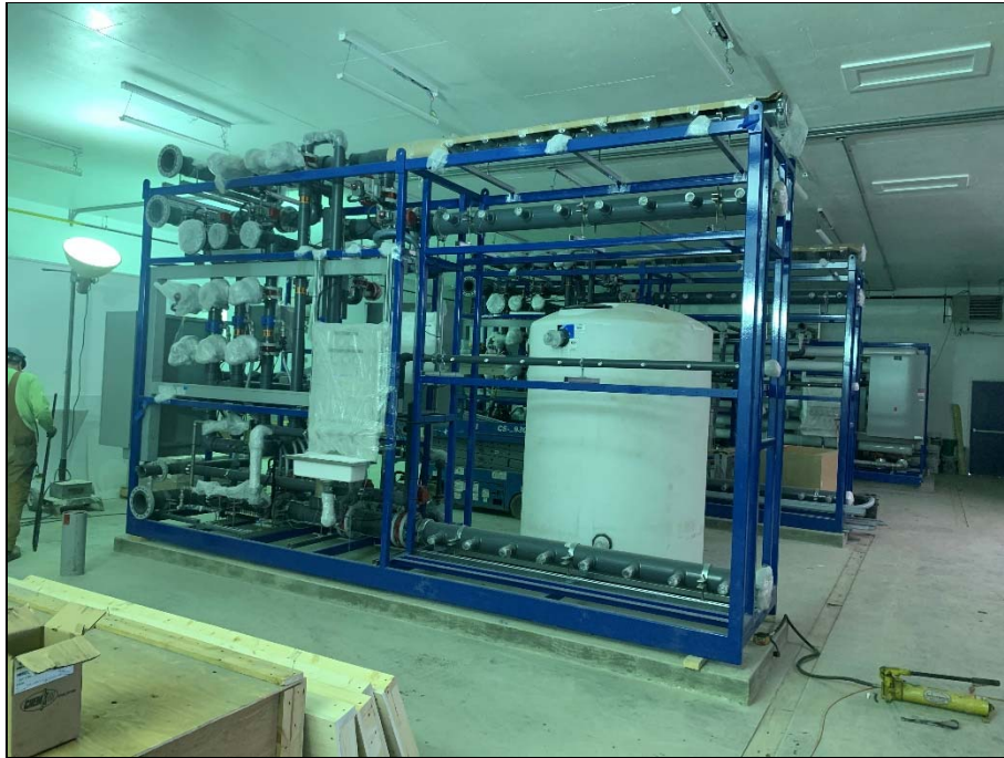
Ultrafiltration (UF) skid no. 1 in place; UF no. 2 (behind) is next to be set.
