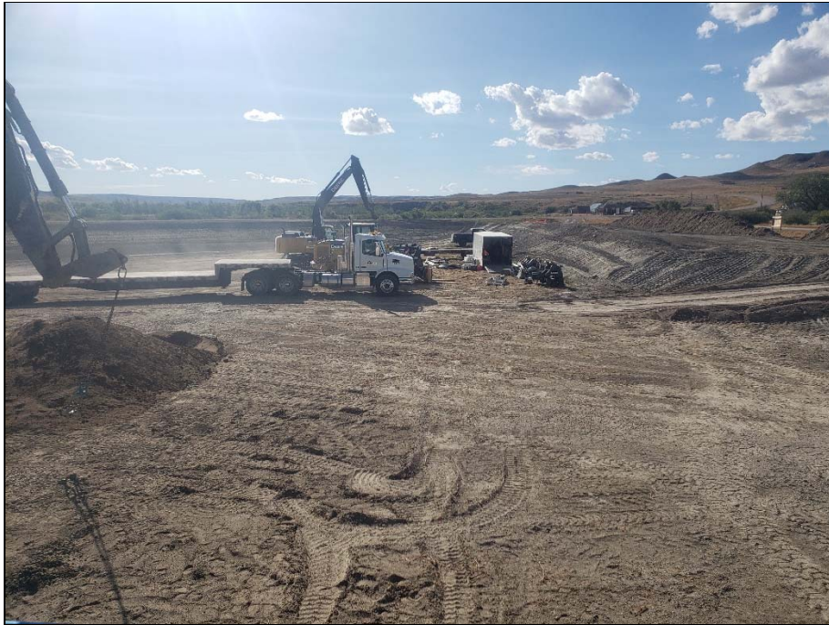
Imported material to build up berms of the raw water reservoir (pond).
