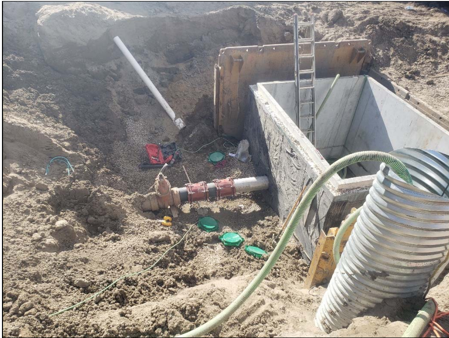
River intake structure and intake line.
