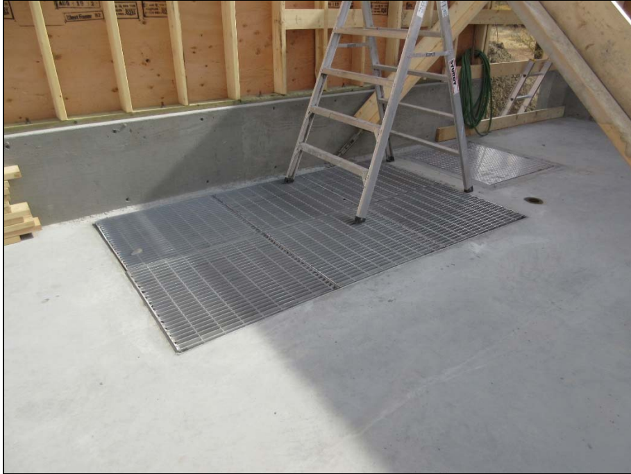
Dry pit access frames.
