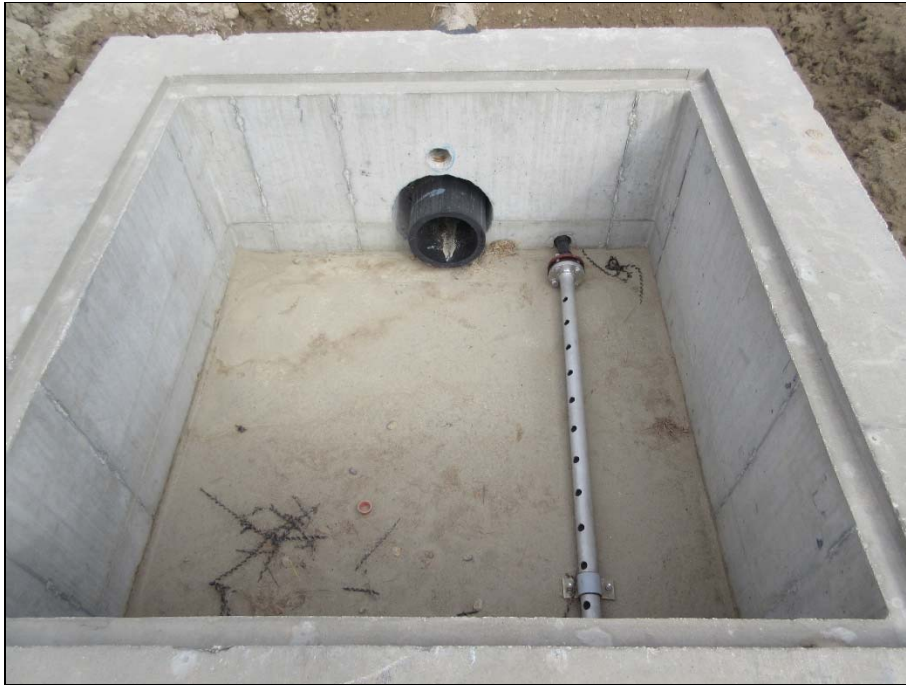
Reservoir intake structure (grating yet to install) with air scour / hot water line.
