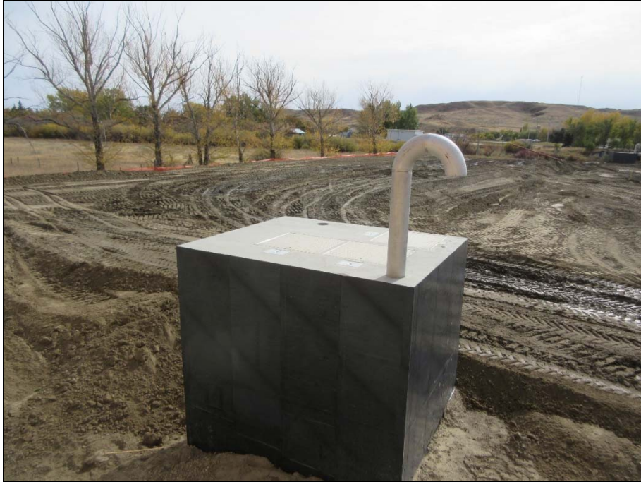
Reservoir intake pumphouse with top slab incl. access hatches, gooseneck vent.
