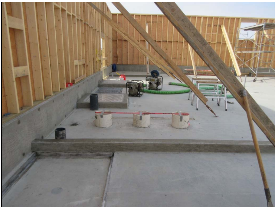
Grating frame, curbs, pump sleeves and access hatches.
