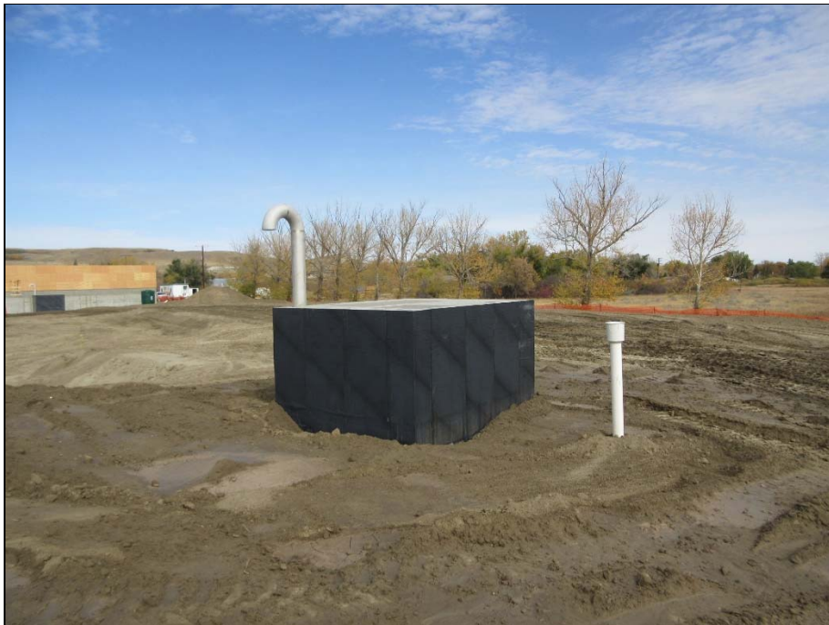
River intake pumphouse.
